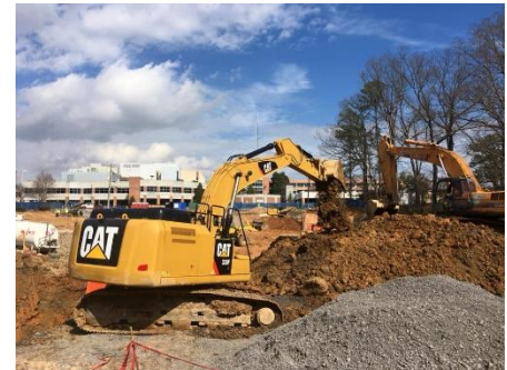
Construction of the newest addition to Hamilton Medical Center, The People's Cancer Institute
