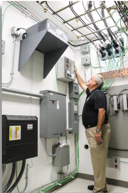
Figure 61: Claude Craig, Emergency Management Director, showcases the County's newest state of the art emergency communications infrastructure enabling emergency responders with reliable communication abilities purchased with previous SPLOST funds.
